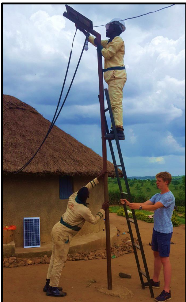
Christian from Germany supporting UE solar technicians to mount a solar panel.
