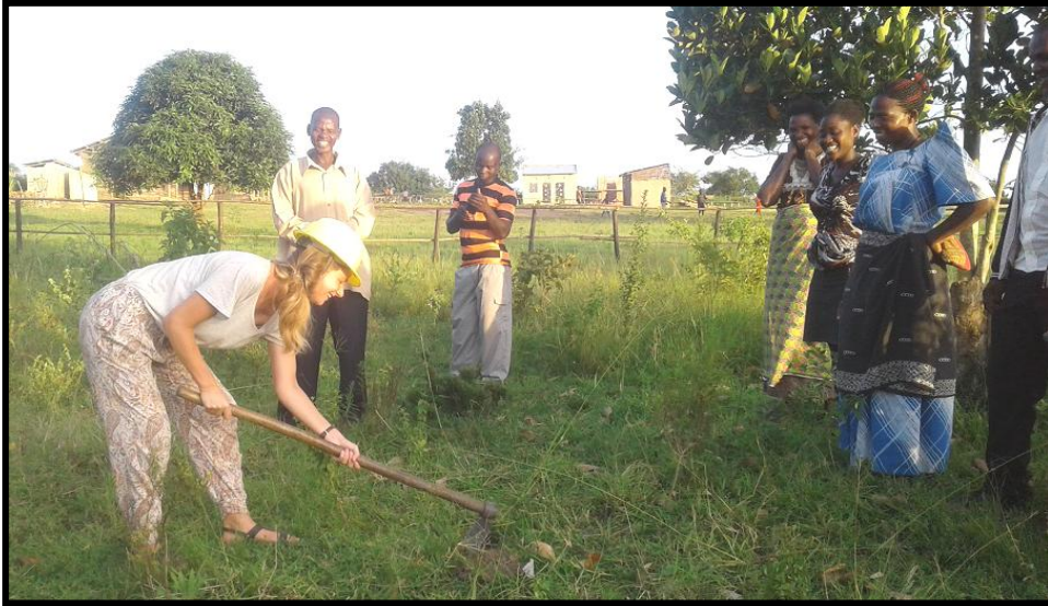
In front of the school management council, Jael doing a ground-breaking to lay foundation for the teacher's house.
